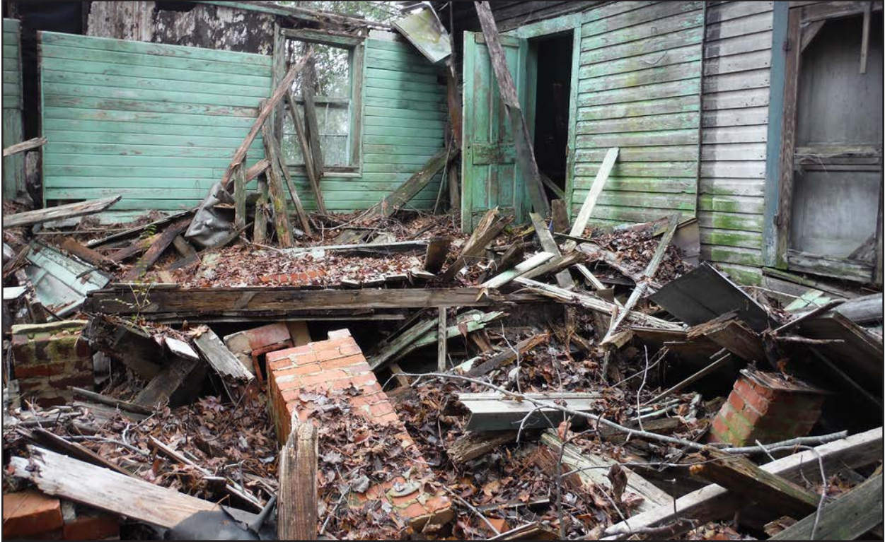
Photo 57. HX1597, dwelling, collapsed addition, facing south.
